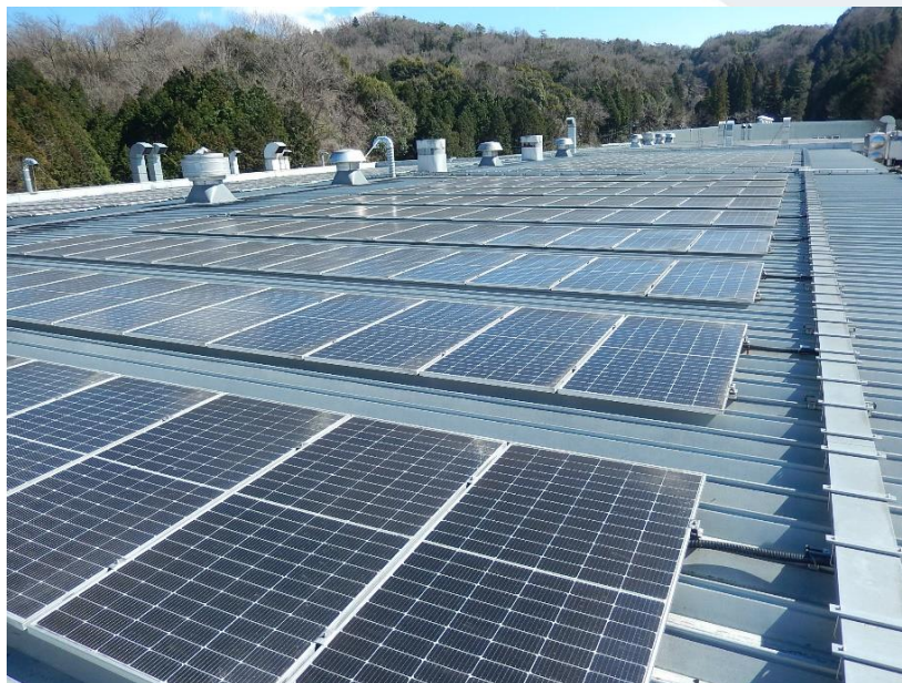
Solar panels installed at Tokai Chemical Industries, Ltd.
